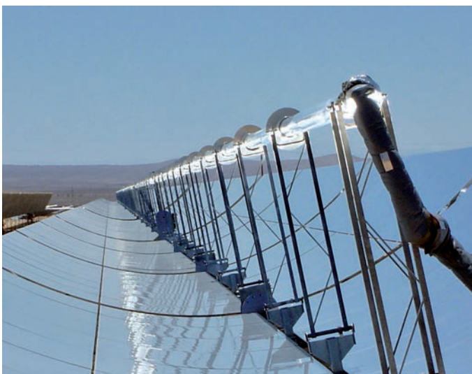
Parabolic Trough Power Plant, Photo: Schott AG
