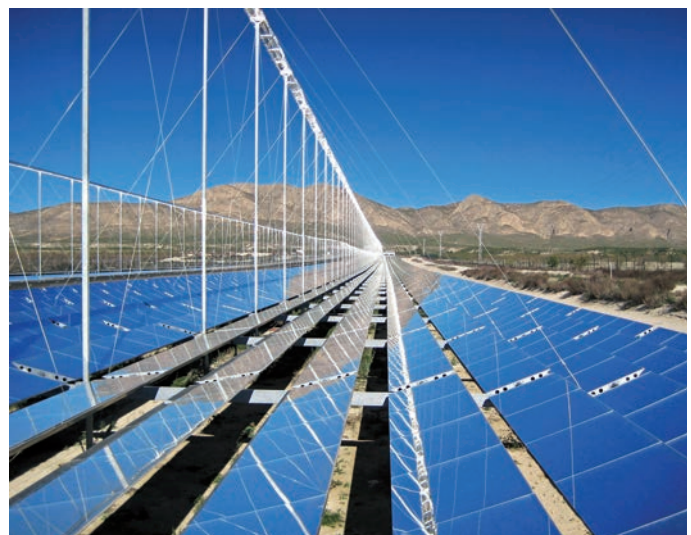
Fresnel Power Plants, Photo: Novatec Solar GmbH
