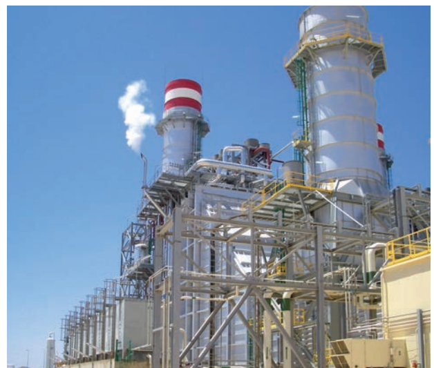
Power Plant, Photo: Schubert & Salzer
