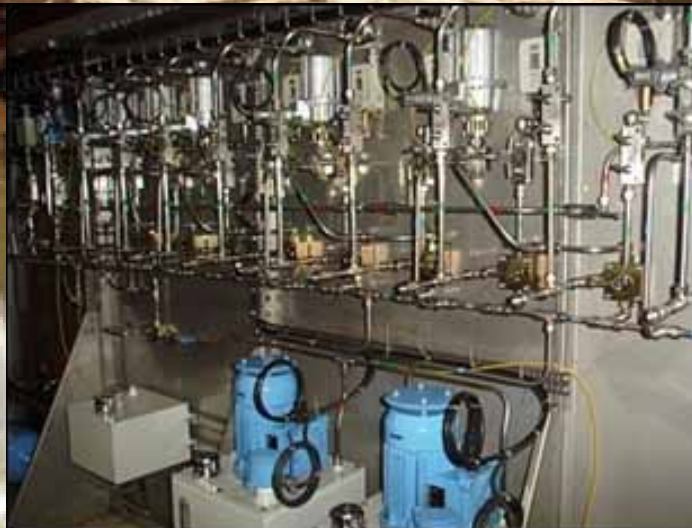
Electric-hydraulic control panels for safety valves 06999.
